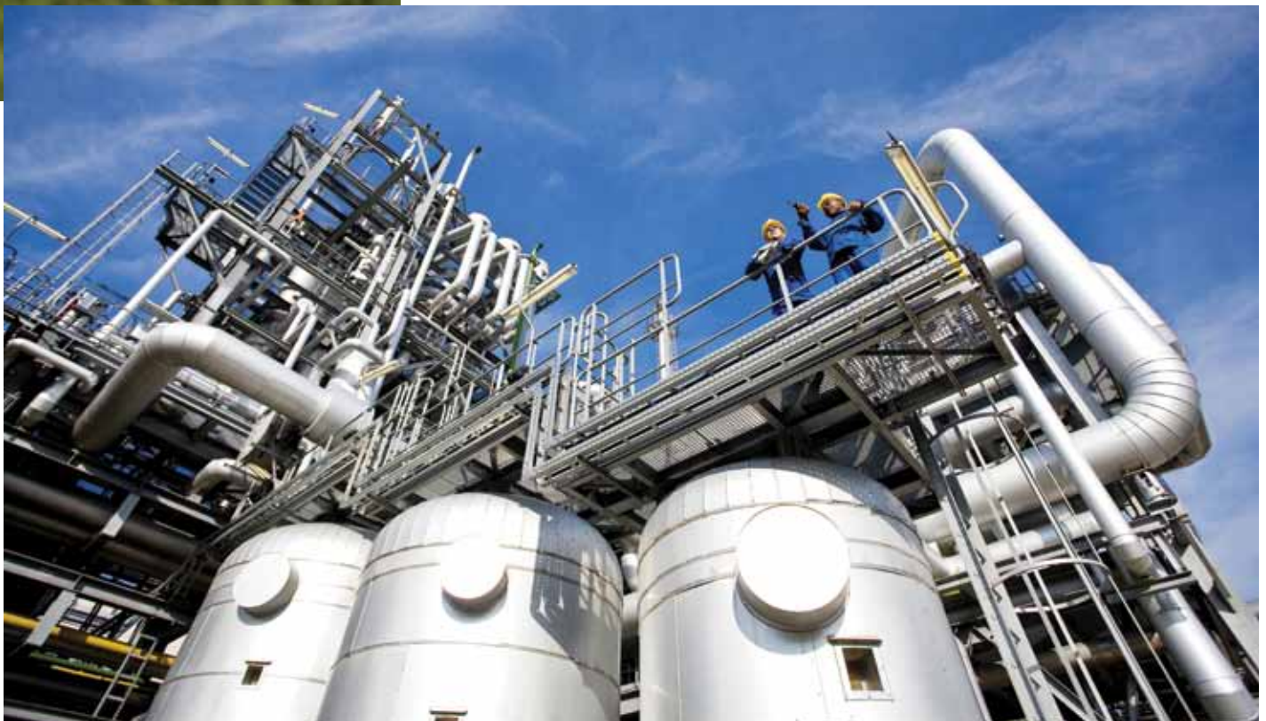
The hydrogen plant at BASF's Verbund site in Ludwigshafen produces hydrogen from natural gas and water vapour in a multi-step process. Excess heat from individual process stages is also used to create steam and feed this into BASF's pressurized (40 bar) network. Photo courtesy BASF SE.
